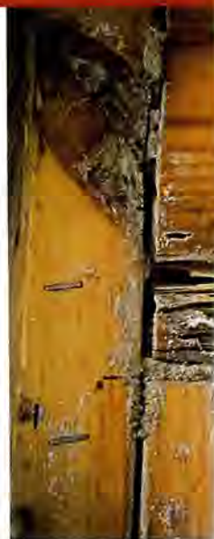
This garage header beam has such an active termite infestation that a pen easily slips through.
